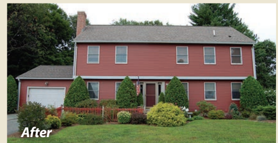
A second-story modular addition doubled the square footage of this ranch home.
